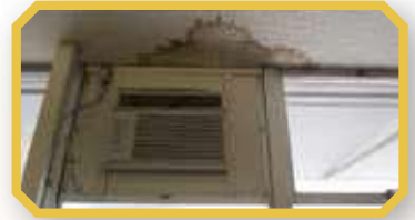
Leaky roofs damage classrooms and disrupt class.
